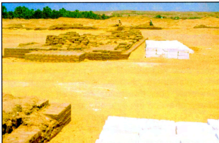
Small Aten Temple – Second pylon entrance. Originally the doorway between the pylon towers was paved with limestone blocks. The plan is to relay the floor with new limestone blocks of a similar size to that of the ancient ones.
